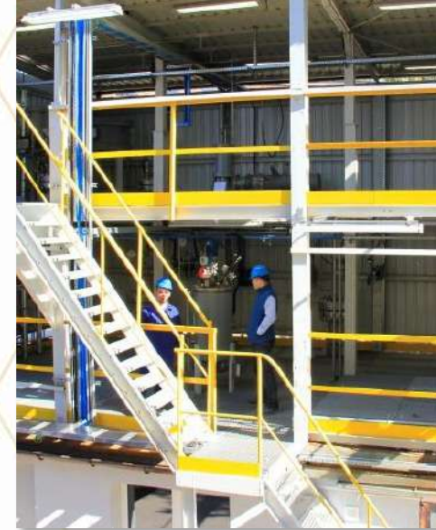
Quarter-technical installation of hydrogen processes
